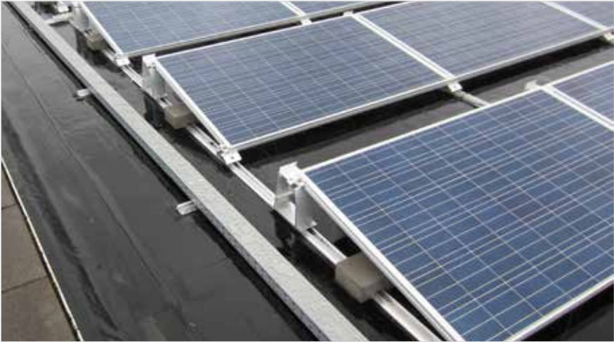
Kaiserslautern, Germany Installation: 2,8 MW | S-Dome System
