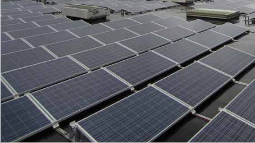
Kaiserslautern, Germany Installation: 2,8 MW | S-Dome System
